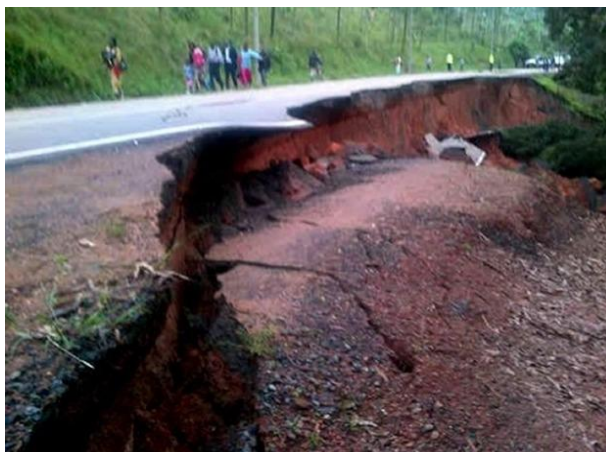
Figure 9: On May 4, 2013, a landslide sliced off a section of the road at Gashenyi Sector in Gakenke district, affecting transport between Kigali and Musanze District.
