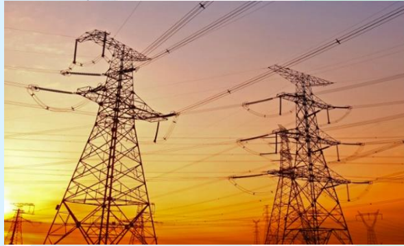
Figure 20: High-tension Transmission line networks
