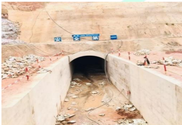
Figure 12: Underground tunnel for river diversion during the construction of the Nyabarongo II Hydropower dam.
