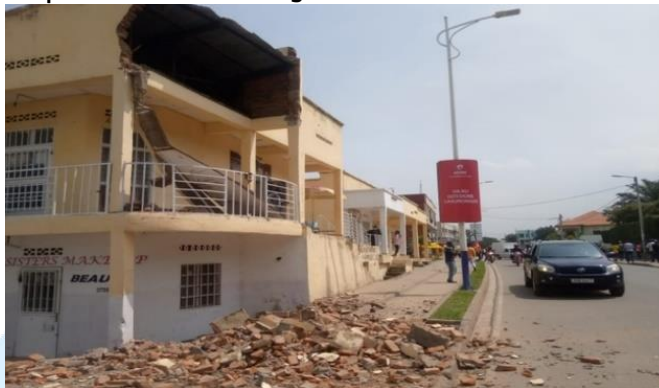
Figure 11: One of the houses damaged by an earthquake in Rubavu in 2021
