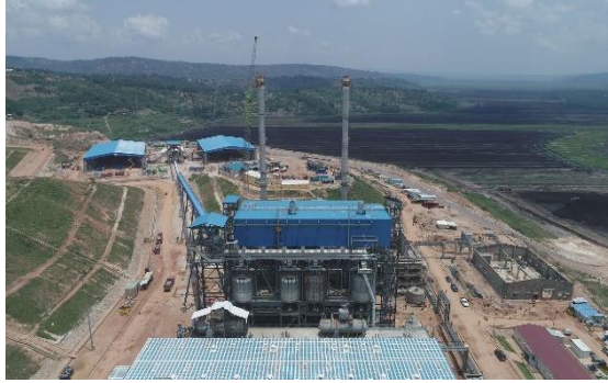
Figure 19: 70 MW peat-fired power plant in Gisagara district
